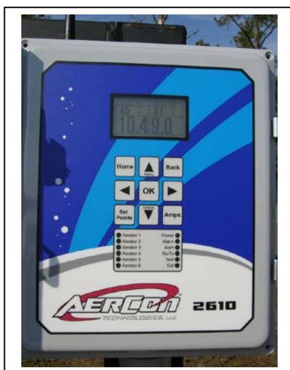
Figure 11 Control box for DO meters. 1
