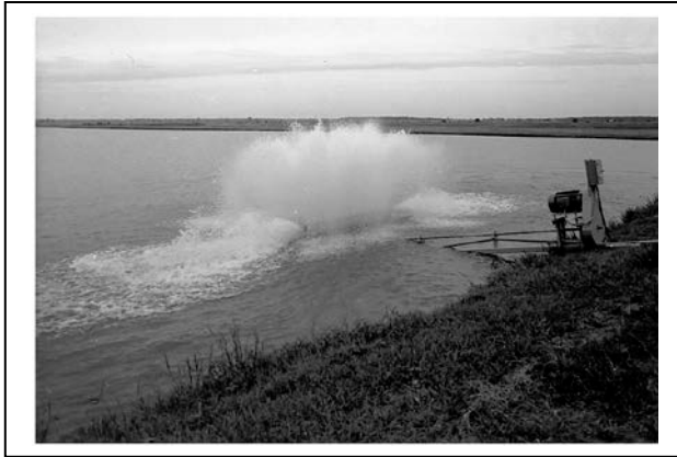
Figure 5 Pump sprayer aerator in operation.
